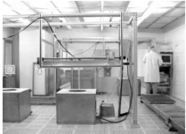
Vertical Laminar Flow HEPA Filter Ceiling
